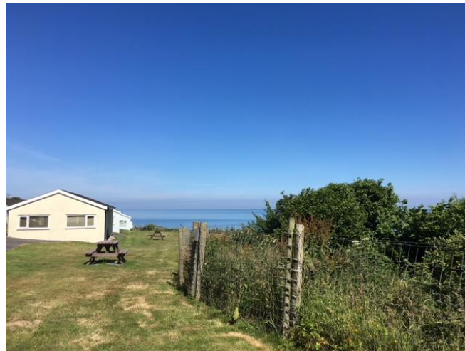
Plate 2. The chalets are proposed for demolition due to erosion of the cliff top upon which they sit.
